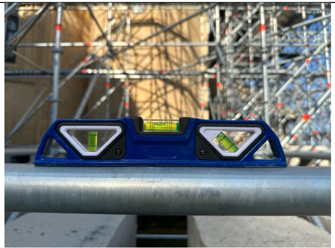
Description: Level Control
