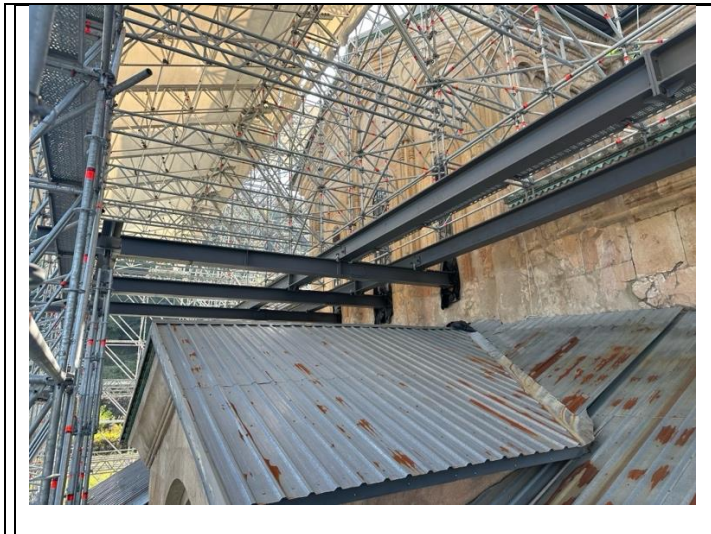
Description: Connection control
