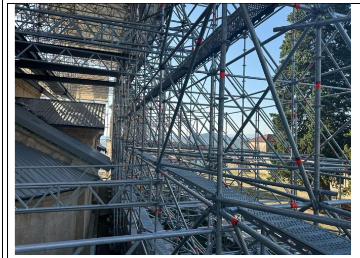
Description: Connection control
