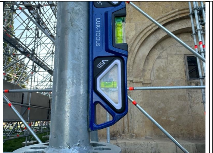
Description: Level Control
