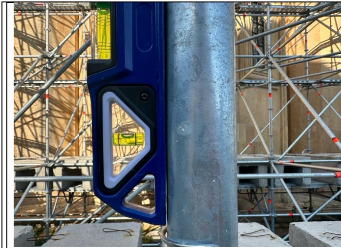
Description: Level Control
