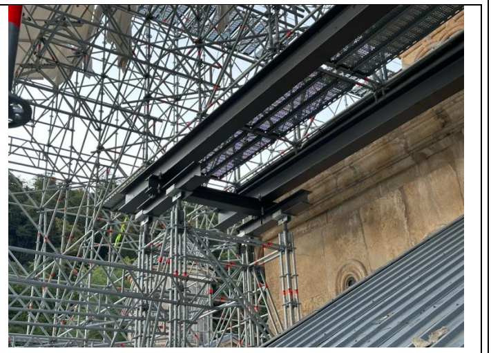
Description: Connection control
