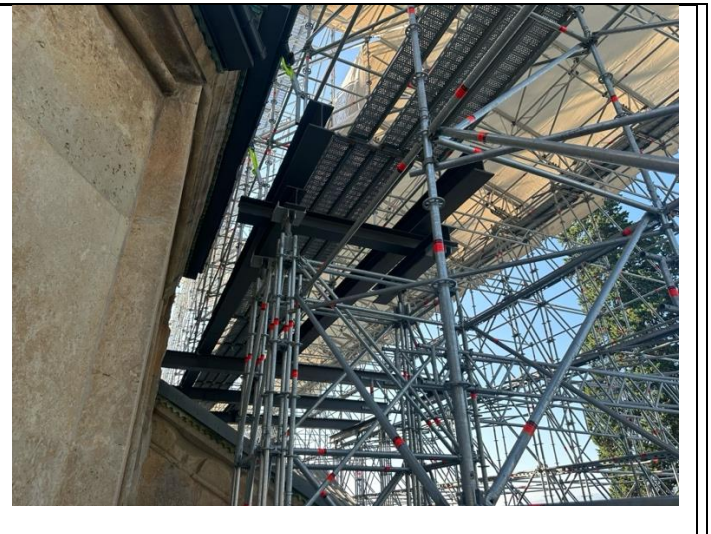
Description: Connection control
