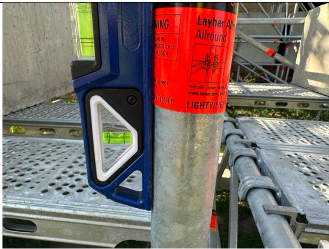
Description: Level Control
