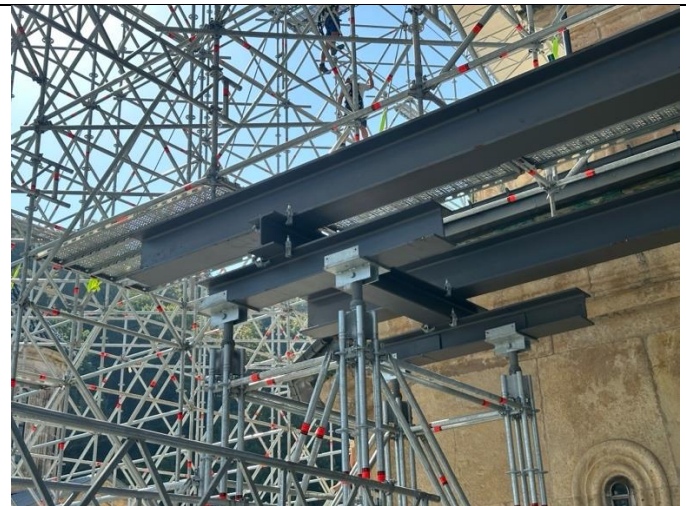
Description: Connection control
