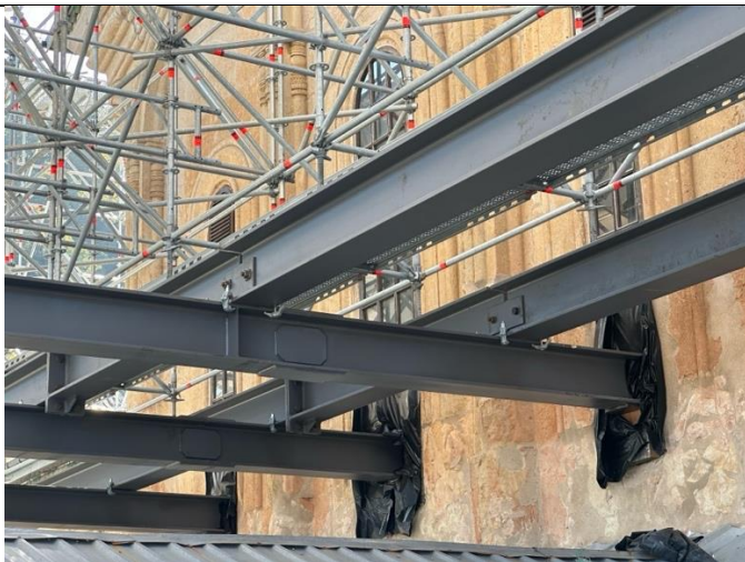
Description: Connection control
