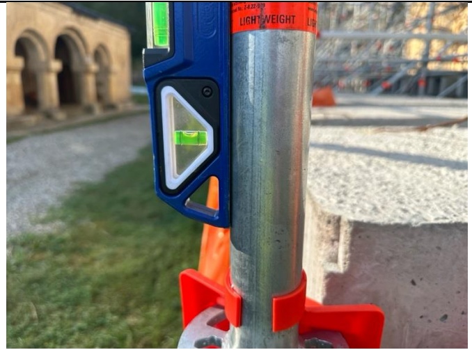
Description: Level Control
