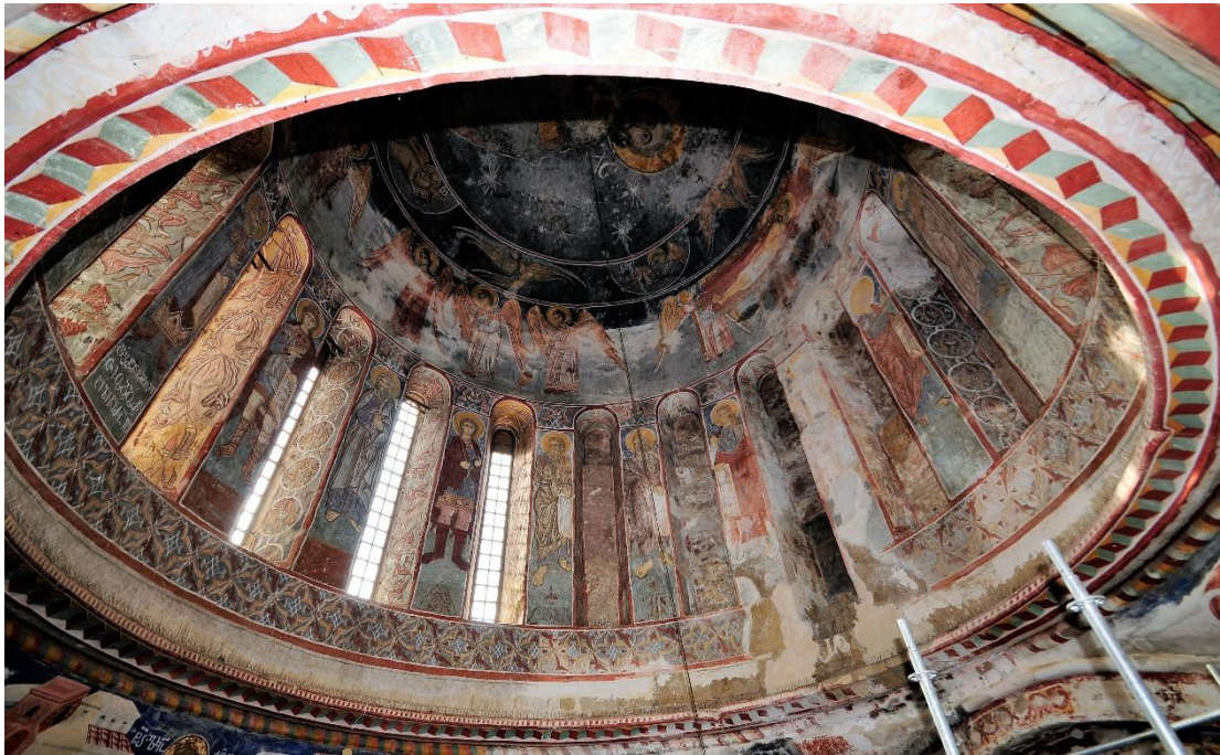
Fig. 1. The drum with visible results of active moisture. The walled window openings on the west side of the tholobate.
