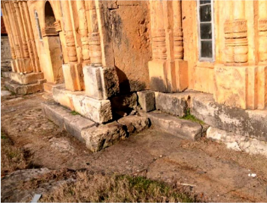
Fig. 16. S-E side: The crepidoma of the Church of the Virgin with the old drainage system around it (2015 joint ICOMOS/World Bank Advisory mission report, fig.10)
