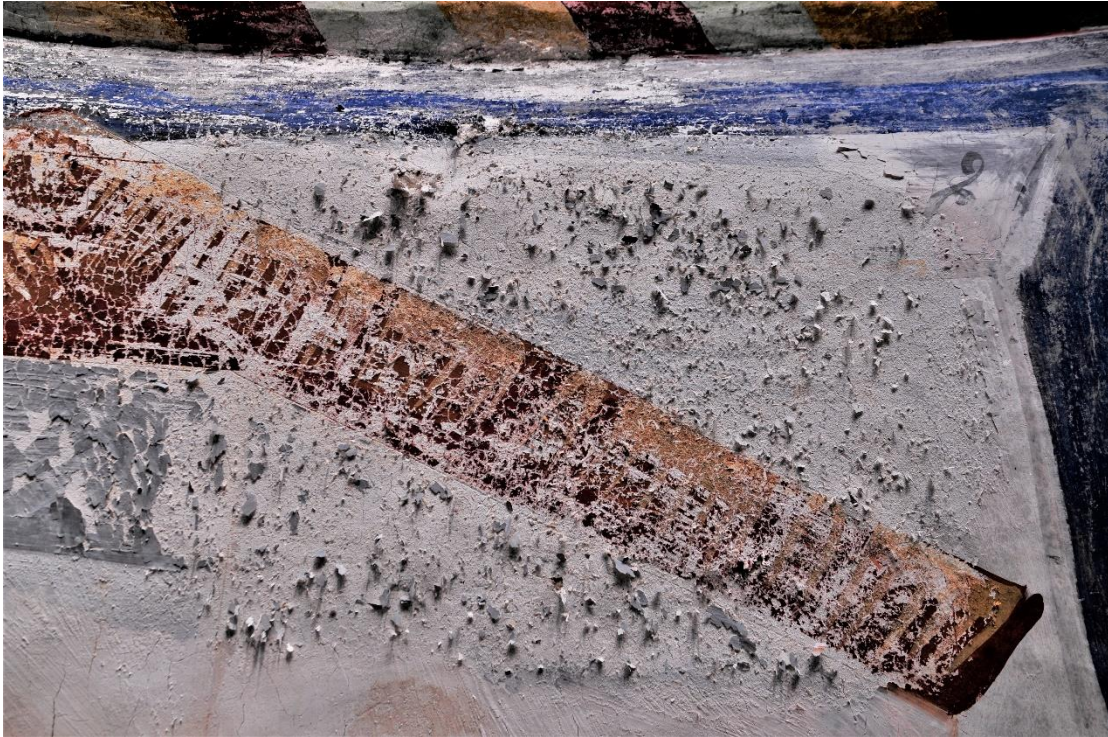
Fig. 8. N-W pendentive: moisture effects.
