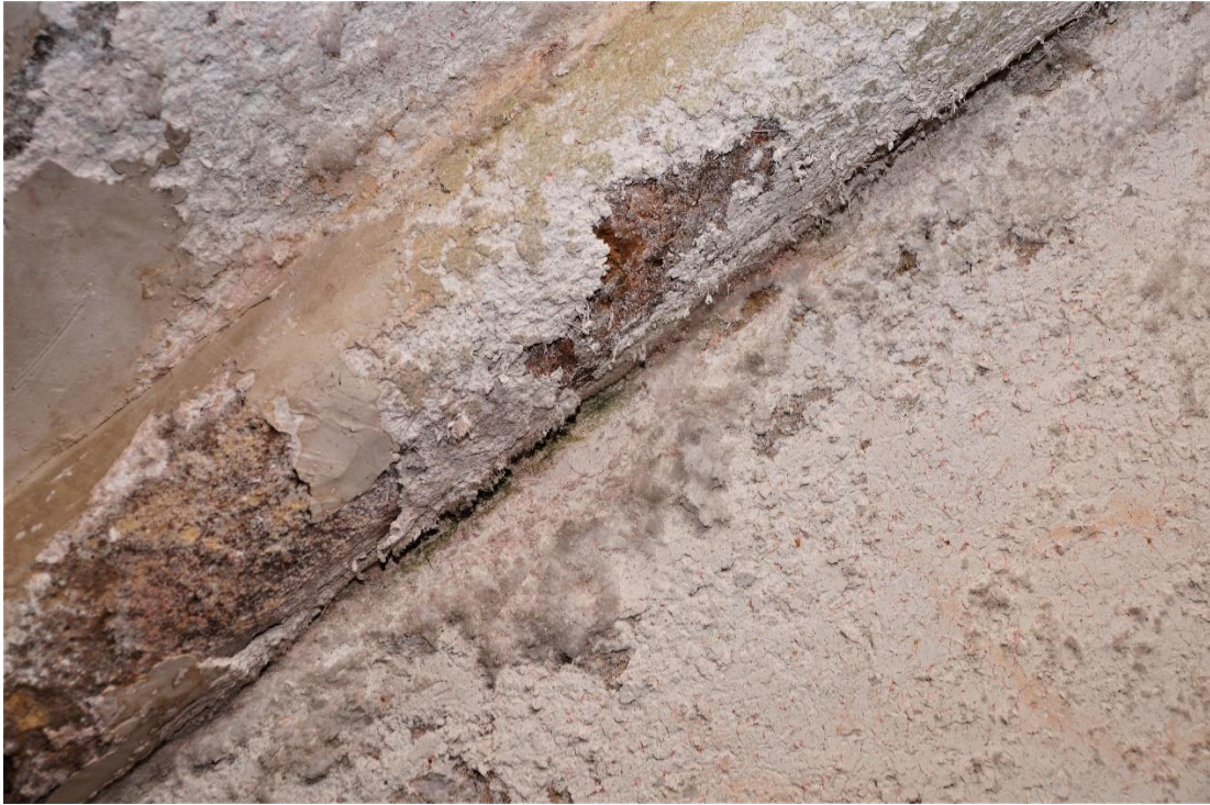
Fig. 6. N-W pendentive: moisture effects.
