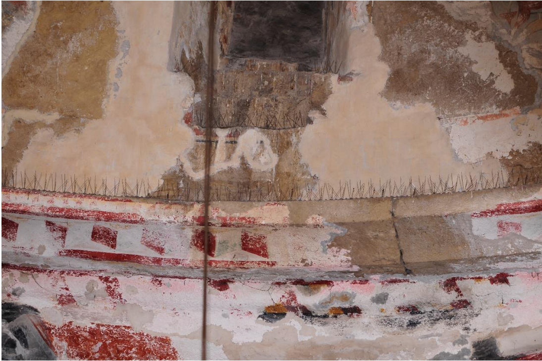
Fig. 4. Drum base west side - the walled exit to outside of the cathedral: old and recent moisture results
