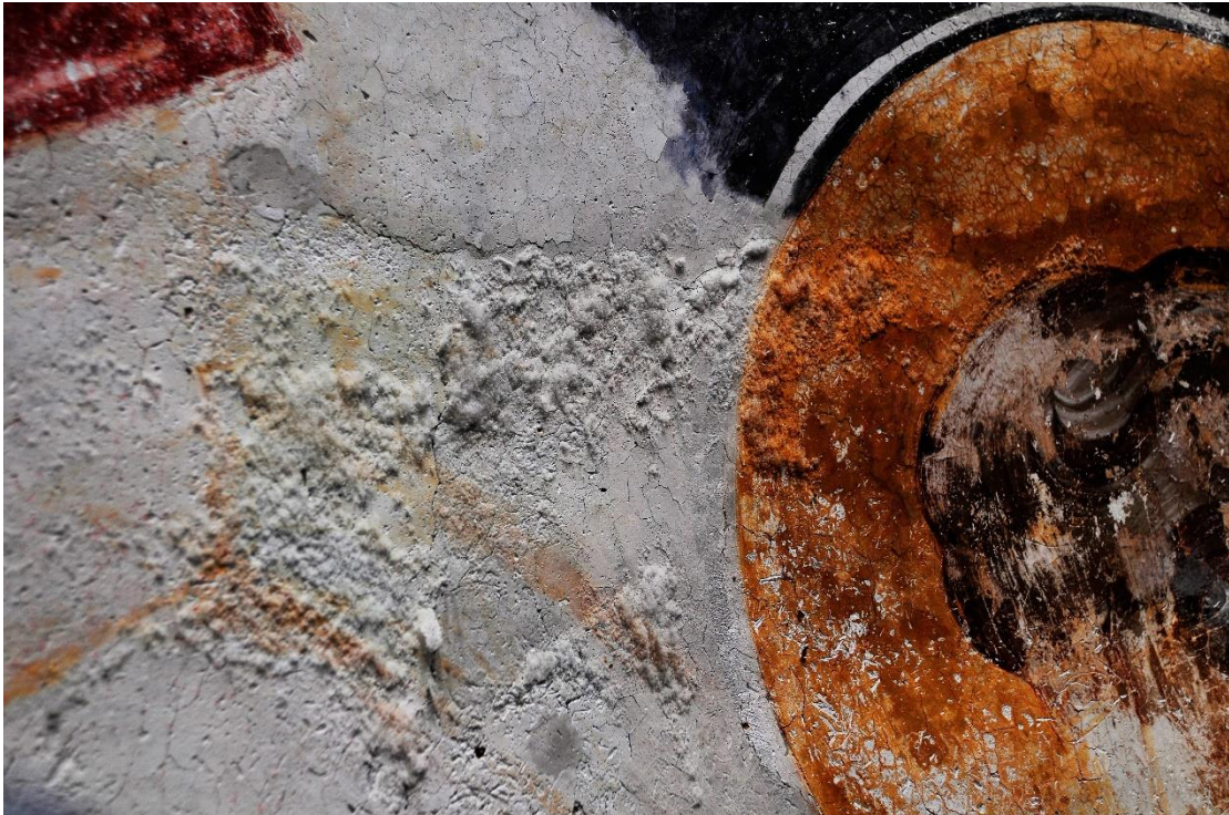
Fig. 7. N-W pendentive: moisture effects.
