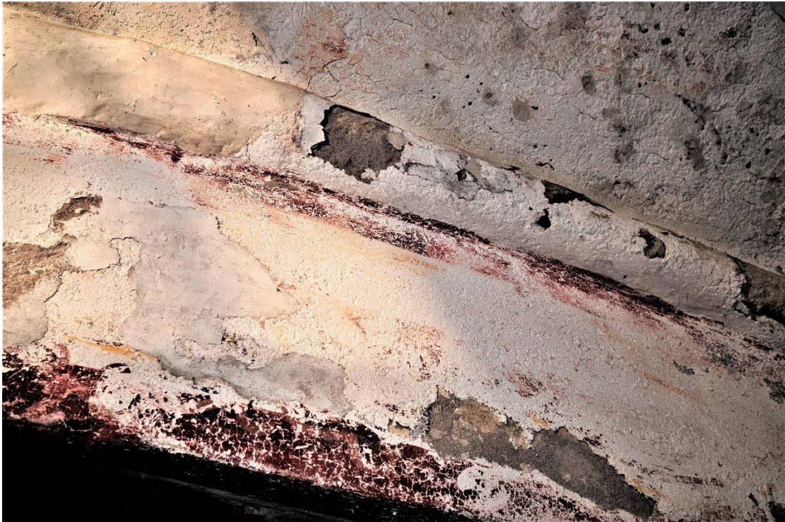
Fig. 5. The ring at the base of drum - west side: moisture effects.
