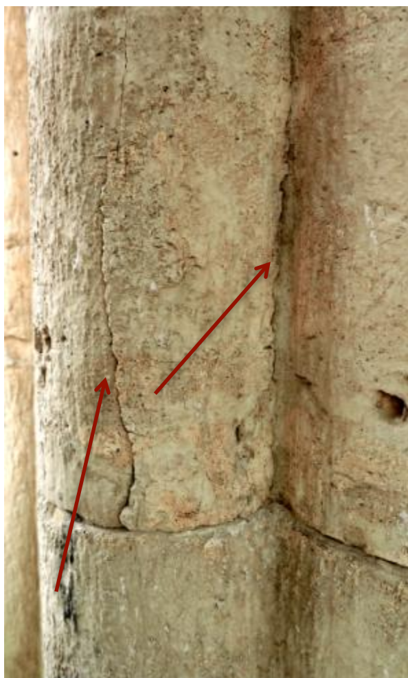
Crackles and fissures caused by contact among ashlars.
