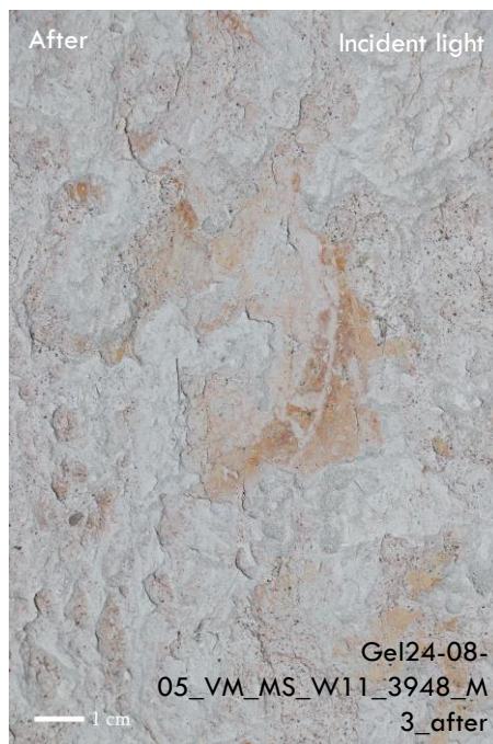
Above: In August 2024, the 2nd phase of remedial treatment programme was undertaken – development of intervention methodologies continued. Plaster consolidation and micro-grouting for securing the exposed plaster edges.
