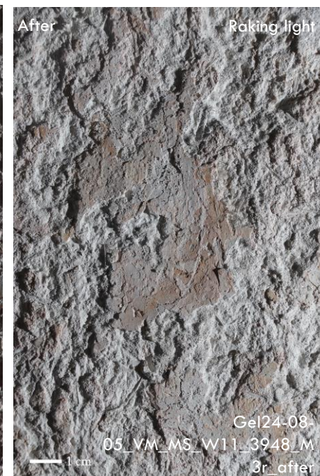
Above: In August 2024, the 2nd phase of remedial treatment programme was undertaken – development of intervention methodologies continued. Plaster consolidation and micro-grouting for securing the exposed plaster edges.
