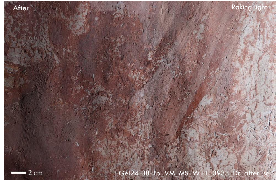
Above: In August 2024, the 2nd phase of remedial treatment programme was undertaken. Paint flakes have been re-adhered using nano-lime consolidant.
