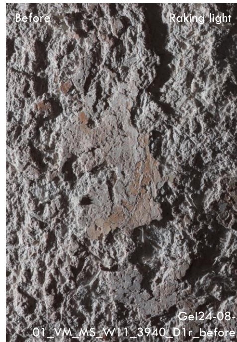
Above: Condition of wall paintings before intervention in August 2024. Plaster delamination, plaster powdering, exposed plaster edges; salt efflorescence
