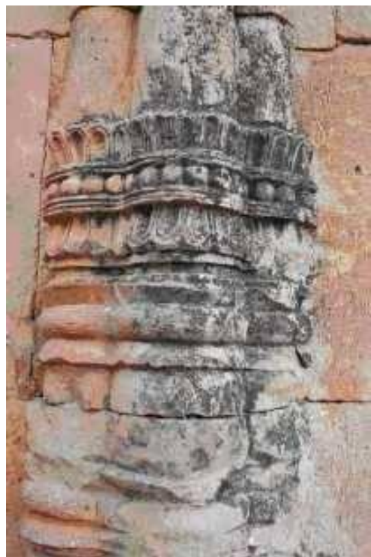
Biological damage of the stone surface
