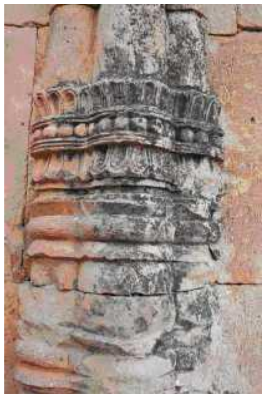
Biological damage of the stone surface
