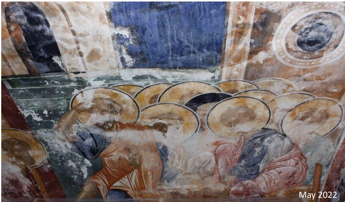
Figure 3a, 3b and 3c. Images of the west arm vault, south side in December 2017, March 2021 and May 2022 show the severity and ongoing nature of the current deterioration due to moisture and salt activity.
