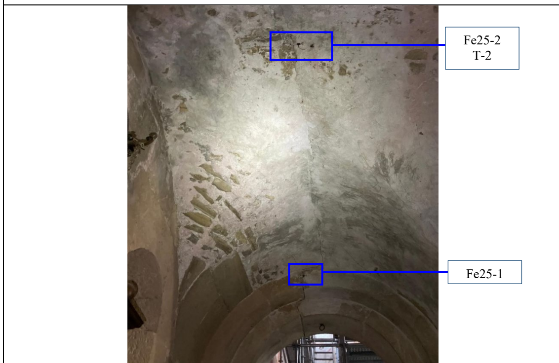
Displacement transducers Fe25-1 e Fe25-2, Temperature sensors T-2 wall.
