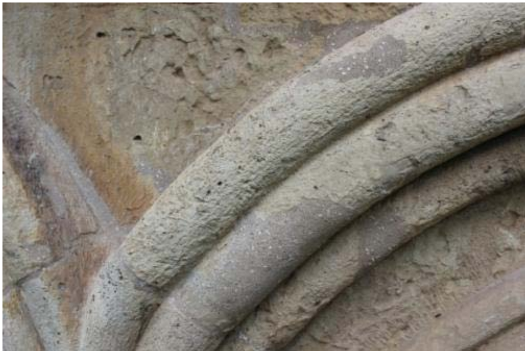
40-41. Consolidation of missed parts of masonry by lime and pozzolana. Northern side
