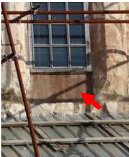
Fill material on the western façade.
