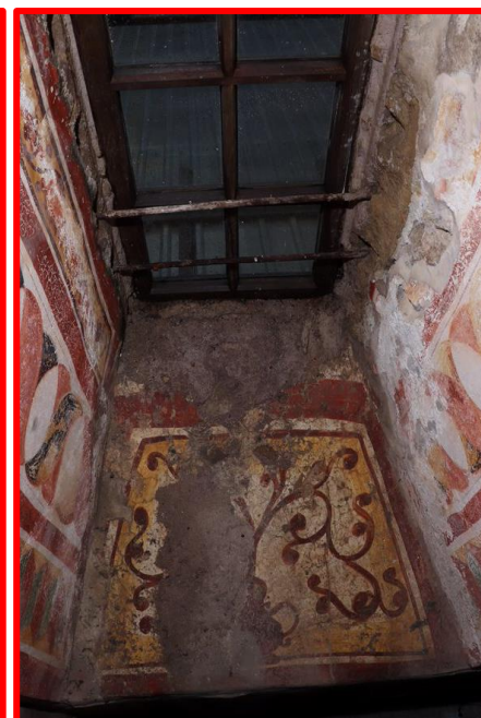
Wet part of the window base, interior.
