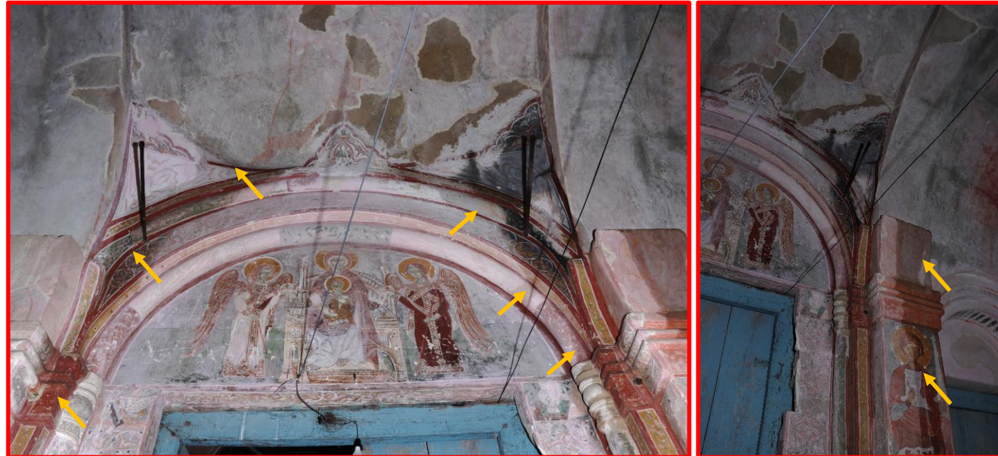
The east wall and vault of the narthex. Locations of water infiltration are marked with yellow arrows.
