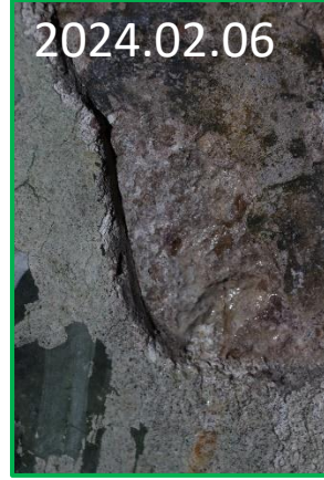
2024.02.06 Left: Scene N6 Church of Virgin, main space, west arm, north wall, water flow.
