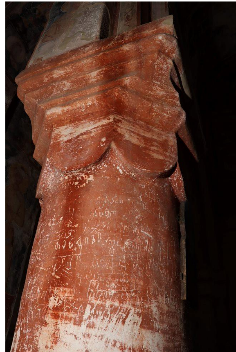
Date of image: 2024.02.08; South-West column, stain of water
