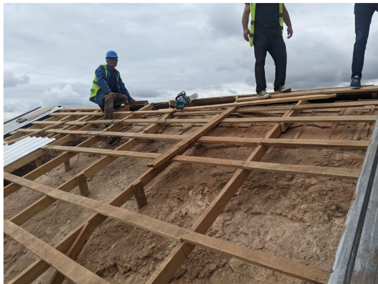
Figure 4. The WA pitch after the removal of the external layers of the roof, and before covering it back with the tin temporary cover (photo by Architect Lasha Shartava).
