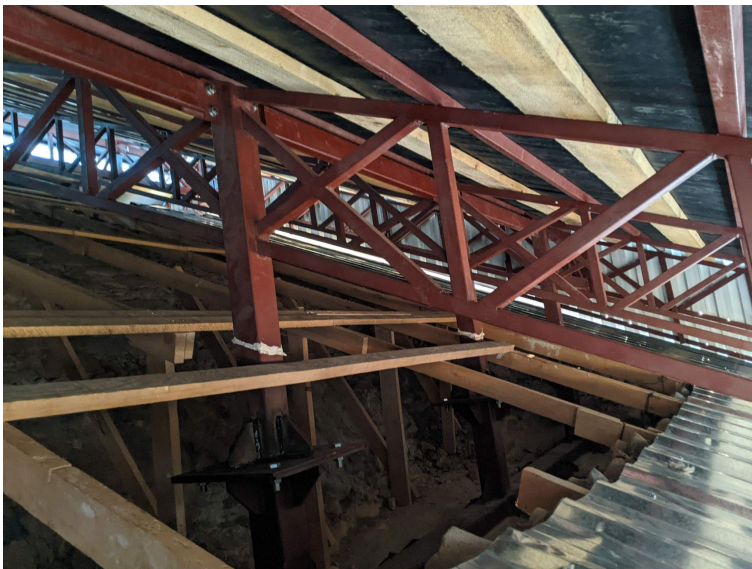
Figure 10. The WA temporary covering, view from the inside (photo by Architect Lasha Shartava).
