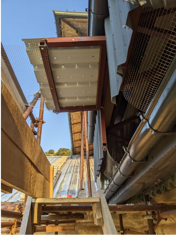
Figure 12. Details of the WA temporary covering: gutter line and opening for internal inspection (photo by Architect Lasha Shartava).
