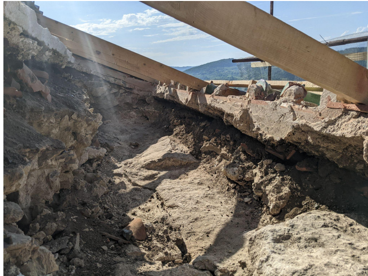
Figure 1. Northern wall of West Arm, clean view of the opening. The longitudinal crack is visible.
