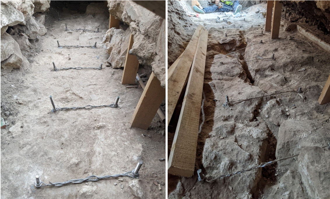
Figure 3. The stitching of the longitudinal cracks on the Northern (left) and Southern (right) walls (photos by Architect Lasha Shartava).
