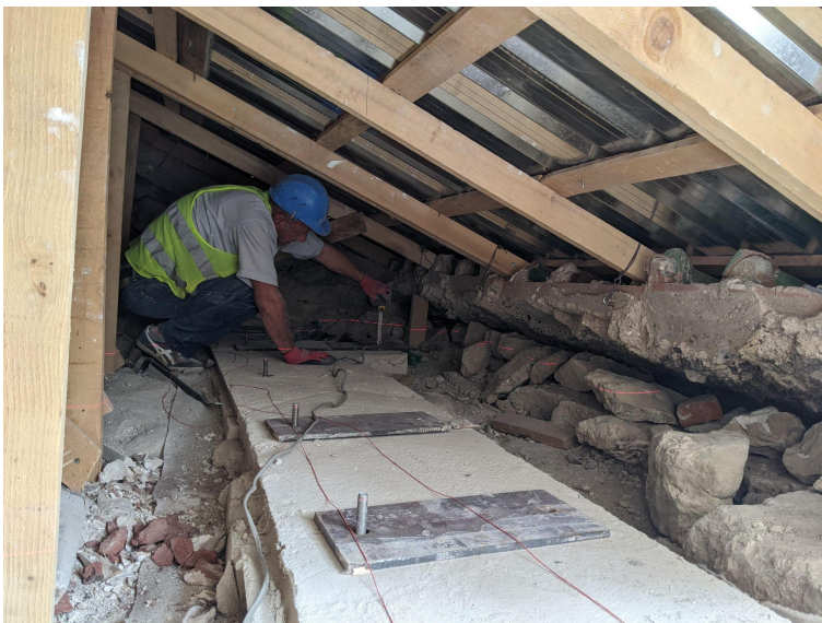
Figure 5. The lime levelling layer for the anchoring and operations to install the anchors of the temporary cover (photo by Architect Lasha Shartava).
