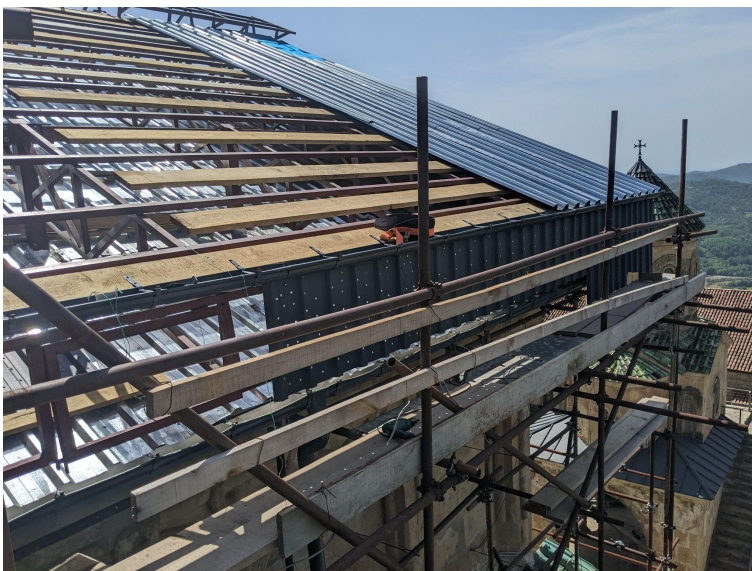
Figure 8. Installation of the tin sheets of the covering and tin sheets with holes to permit ventilation. The perforated sheets are darker to avoid visual impact and glare caused by the reflection of the sun's rays (photo by Architect Lasha Shartava).
