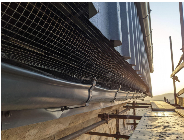
Figure 11. Details of the WA temporary covering: gutter line (photo by Architect Lasha Shartava).
