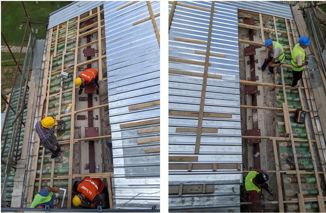
Figure 6. The anchoring of the temporary cover for both pitches (photos by Architect Lasha Shartava).
