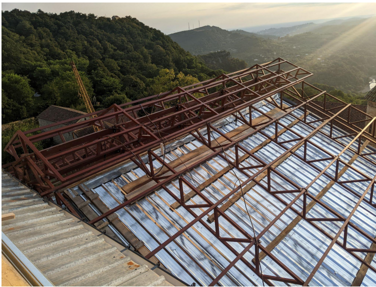
Figure 7. The metal trusses with the pre-fabricated structure on the ridge of the pitches, useful for the chimney effect (photo by Architect Lasha Shartava).
