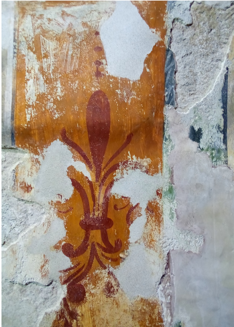
North wall - new stucco filling (stuccature) grouting with lime paste (grassello di calce) mortar and river sand
