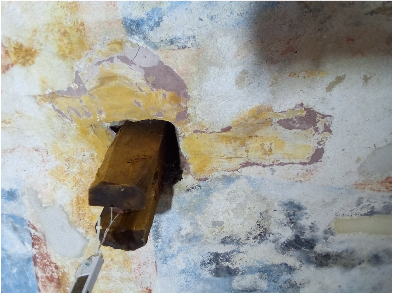
Old unsuitable stucco fillings (stuccature) near the cross
