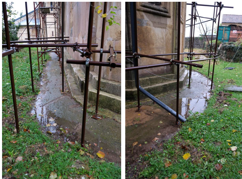
Figures 20 and 21 - Views of water stagnations along the outer perimeter of St. George, particularly abundant along the South and East sides due to water also coming in from the roofs (from MCT SG report).
