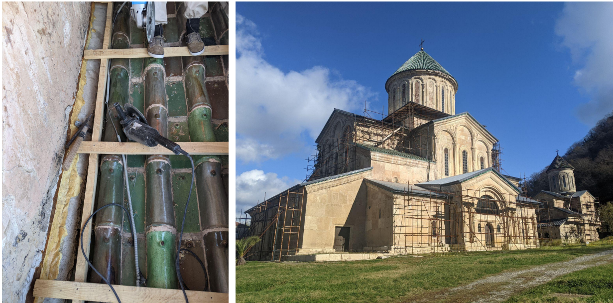
Figure 10 - Absence of flashing at the intersection between the pitch and the vertical wall; Figure 11 - Absence of gutter and downpipes in the Monastery.
