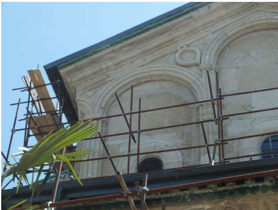
Western wall of West Arm. Cracks on cornices.
