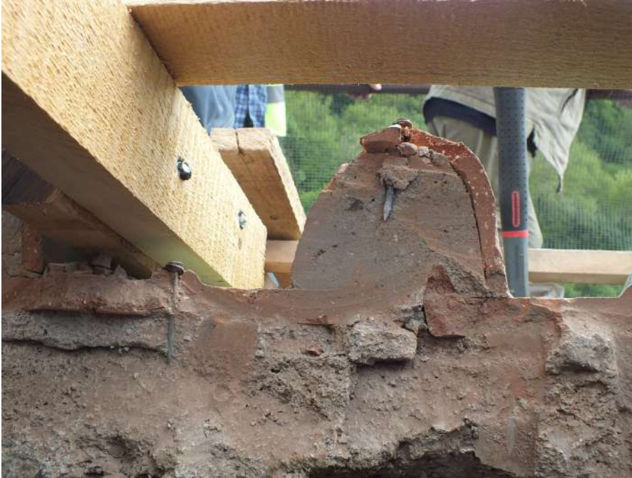
Southern wall of West Arm. Section of the roof layers regarding the last intervention.
