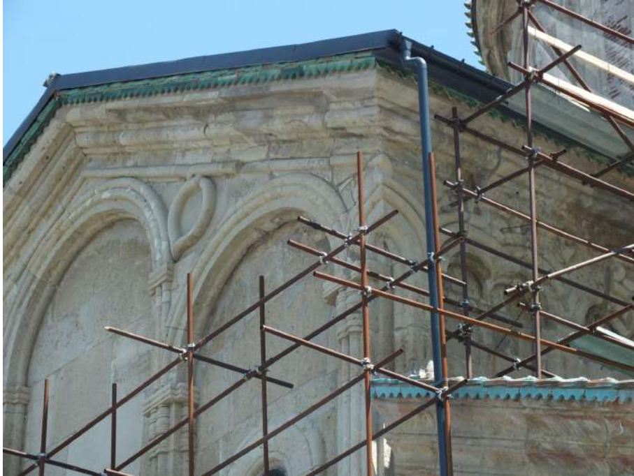
Southern wall of West Arm. Cracks on cornices and arches.
