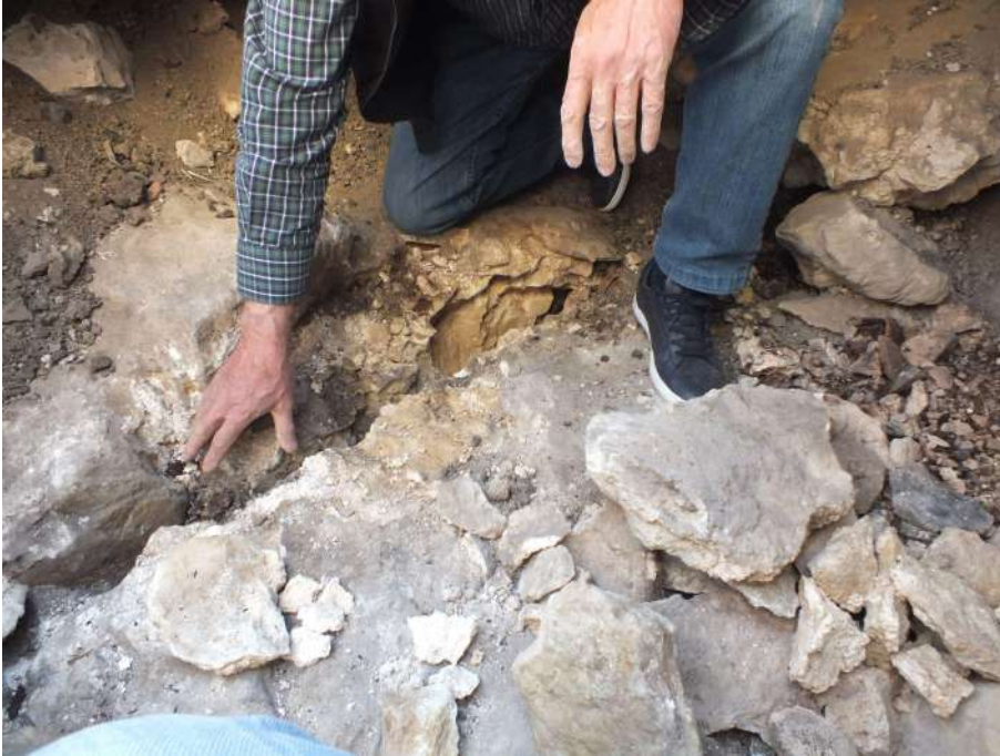
Southern wall of West Arm. Longitudinal crack on the top of the wall.
