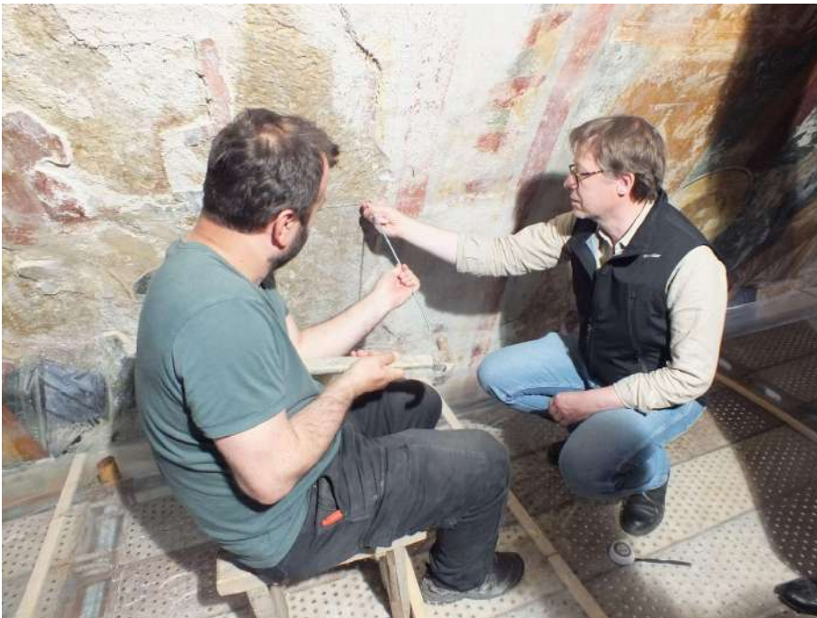
Northern wall of West Arm, interior. Internal-external through hole in the masonry of the vault.
