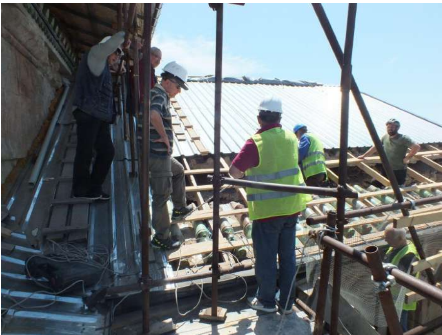
Northern wall of West Arm. Inspection and discussion with Eng. Zurab Okroshidze.
