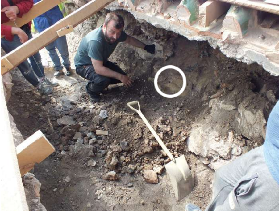
Northern wall of West Arm, extrados. Internal-external through hole in the masonry of the vault.
