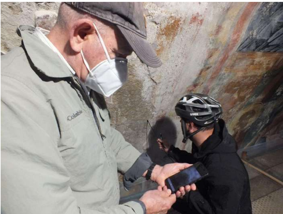
Southern wall of West Arm, interior. Inspection, using an endoscope, in order to check the thickness of the vault.
