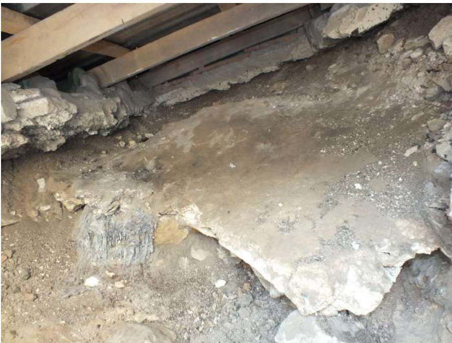
Southern wall of West Arm. The ancient collapsed mortar filling with a molten lead block.
