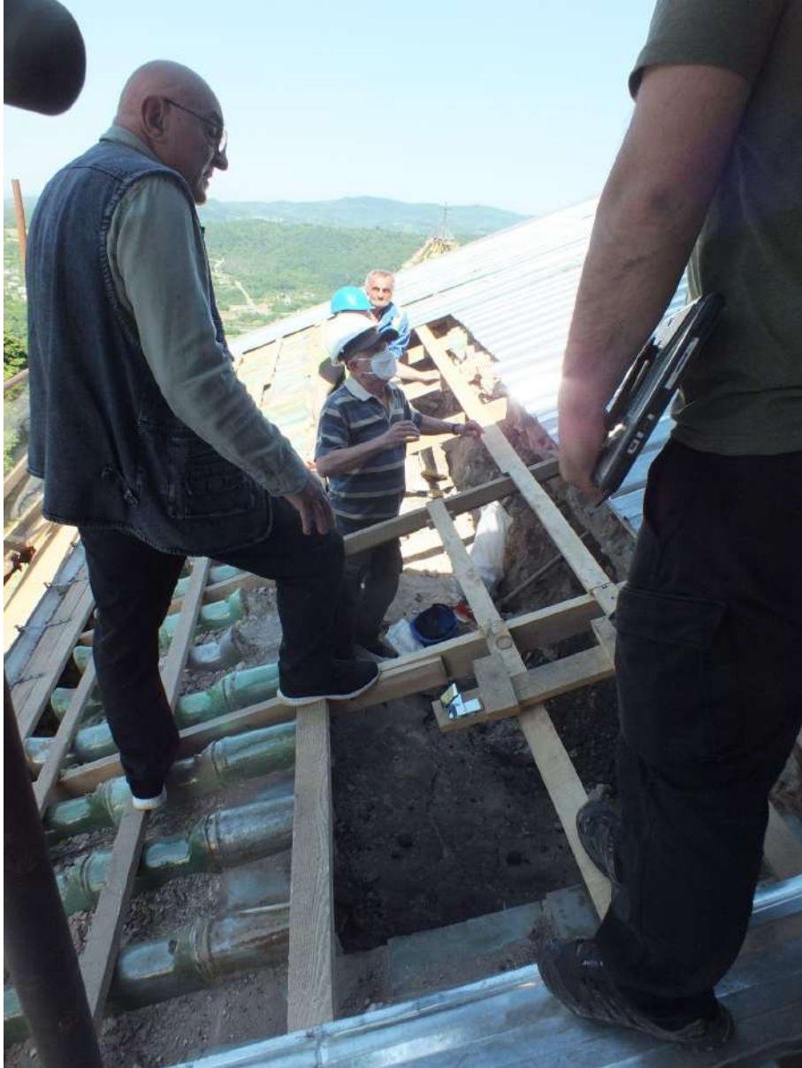
Southern wall of West Arm. Inspection and discussion with Eng. Zurab Okroshidze.
