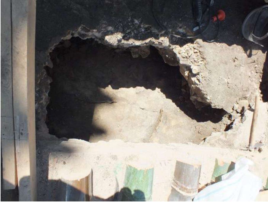
Northern wall of West Arm. Roof opening operations: findings of a longitudinal crack.
