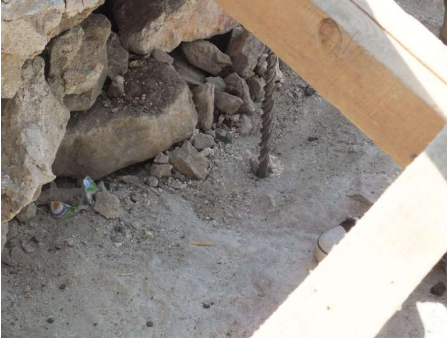
Northern wall of West Arm. Drilling a hole in the core of the wall.
