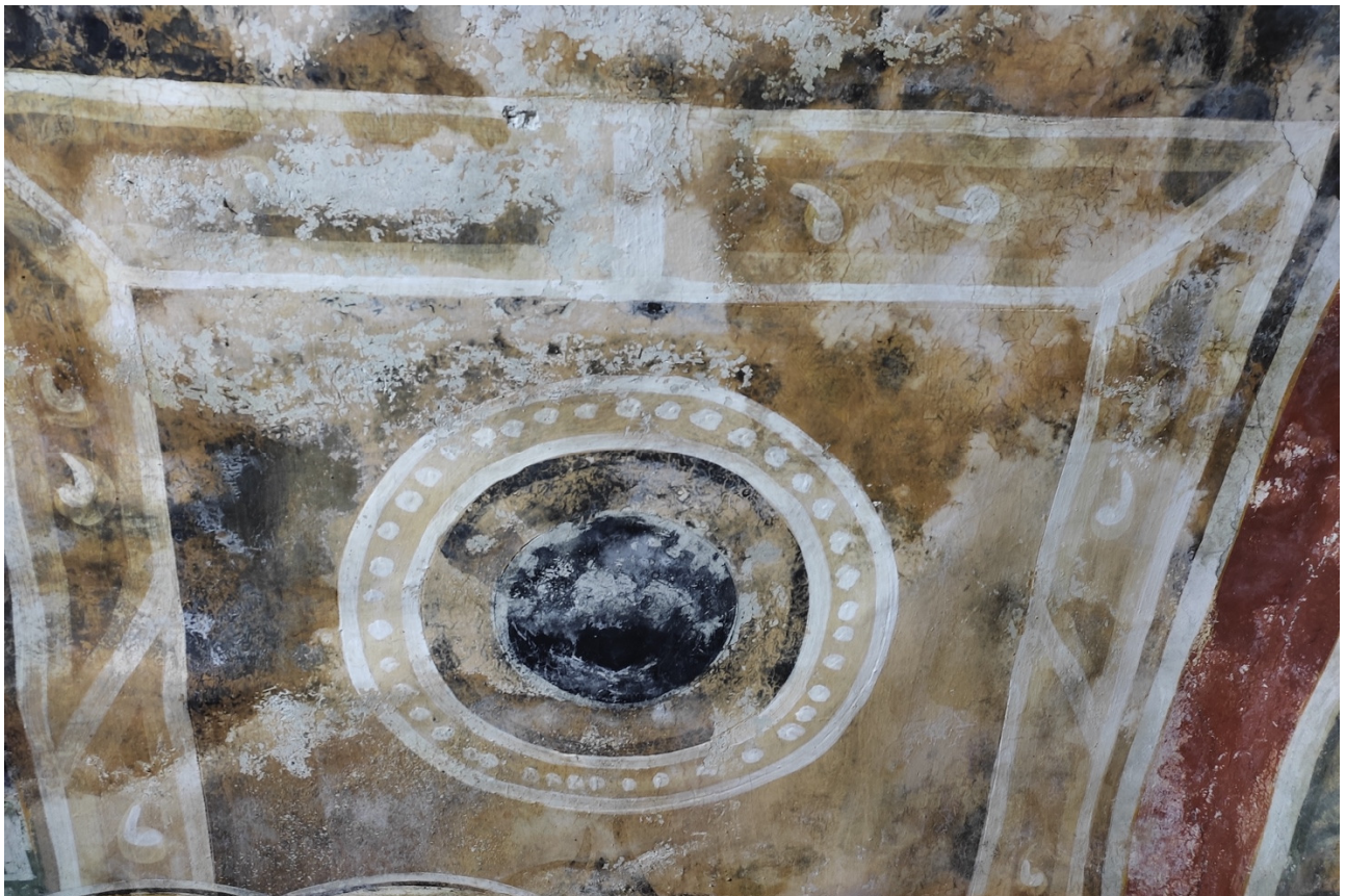
Water stains of humidity much more pronounced
