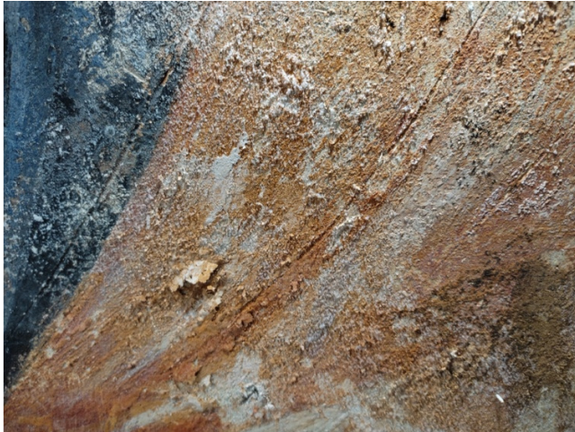
1- new saline efflorescence on the South wall
