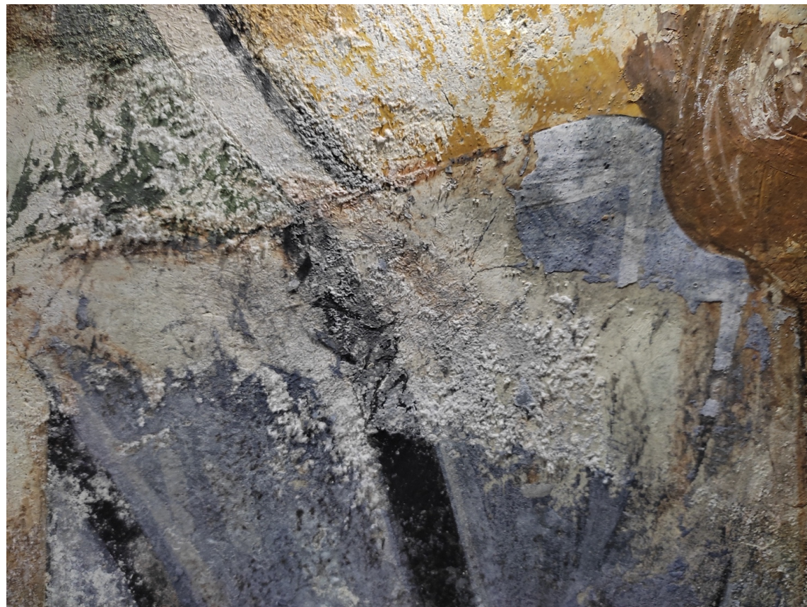
new saline efflorescence on the South wall
