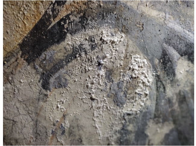
new saline efflorescence on the South wall
