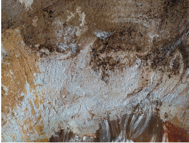
new saline efflorescence on the South wall
