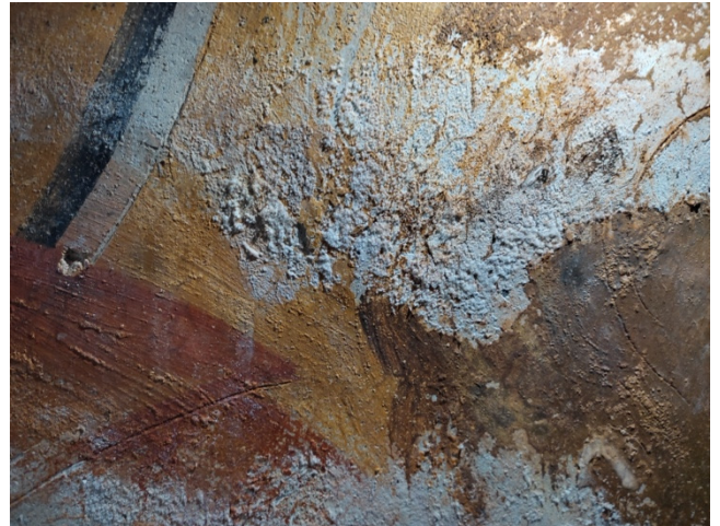
new saline efflorescence on the South wall
