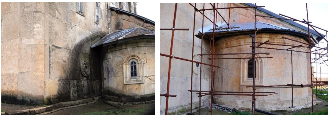
Fig. 55. The N-E apsis of the church to the conjunction with the northern parekklesion (2010 Joint World Heritage Centre/ICOMOS/ICCROM Advisory mission) Fig. 56. The same area during the 2022 Joint WHC/ICOMOS/ICCROM mission
