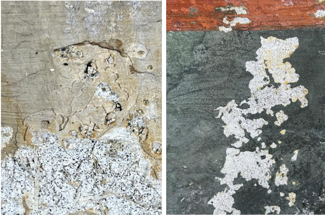
Fig. 27, 28. Subflorescences and paint layer detachment in the southern wall of the west wing
