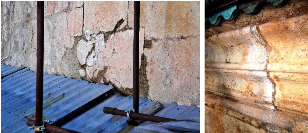
Fig. 51, 52. Condition of the north façade near to north arm – recent humidity on the joints' mortar and salt crystallization
