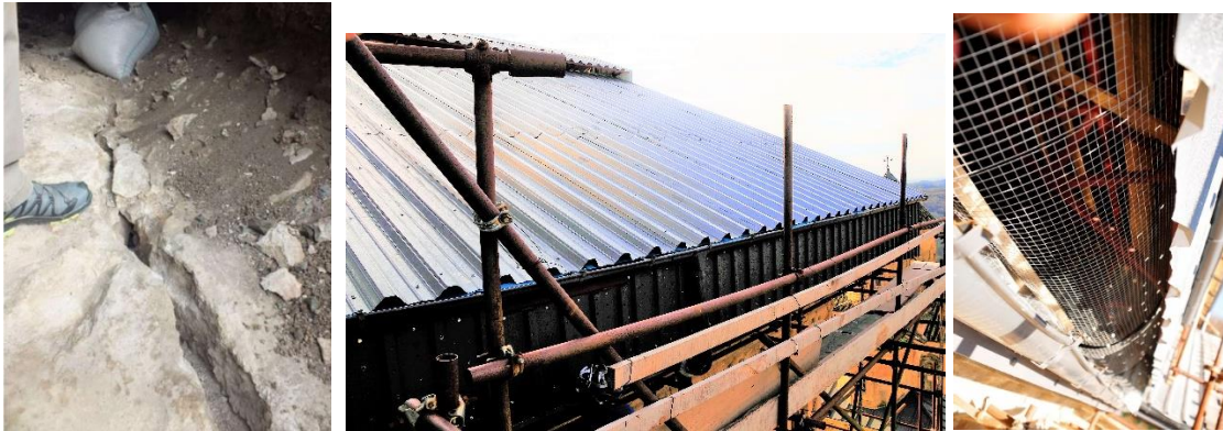
Fig. 20. Southern wall of west arm. Longitudinal crack on the top of the wall (by ReStruere) Fig. 21. West arm, new temporary roofing Fig. 22. Openings allowing air to circulate and facilitating moisture evaporation outside the extrados of the west arm
