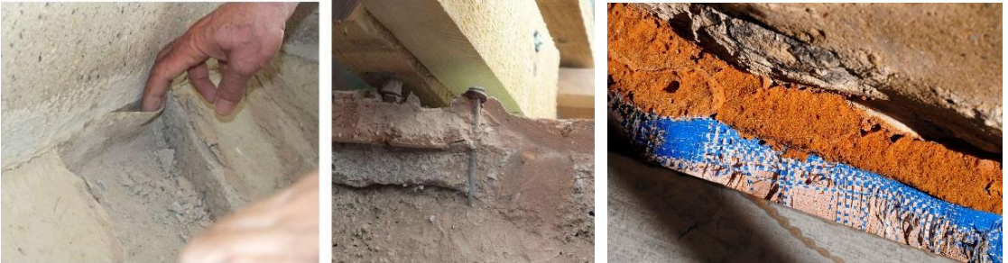
Fig. 12. Incorrect installation technique: a short strip of insulating material / nails penetrating the liquid insulated mortar (by ReStruere)
