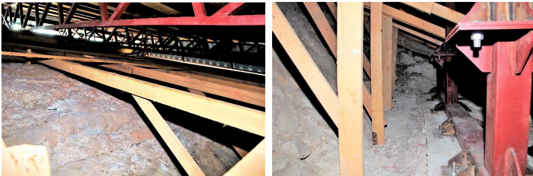
Fig. 23. The iron truss system supporting the new temporary roof covering the extrados of the west arm Fig. 24. The reinforced truss piers supporting the iron truss system, fixed along a concrete base, on the insulated substrate protecting the longitudinal cracks
