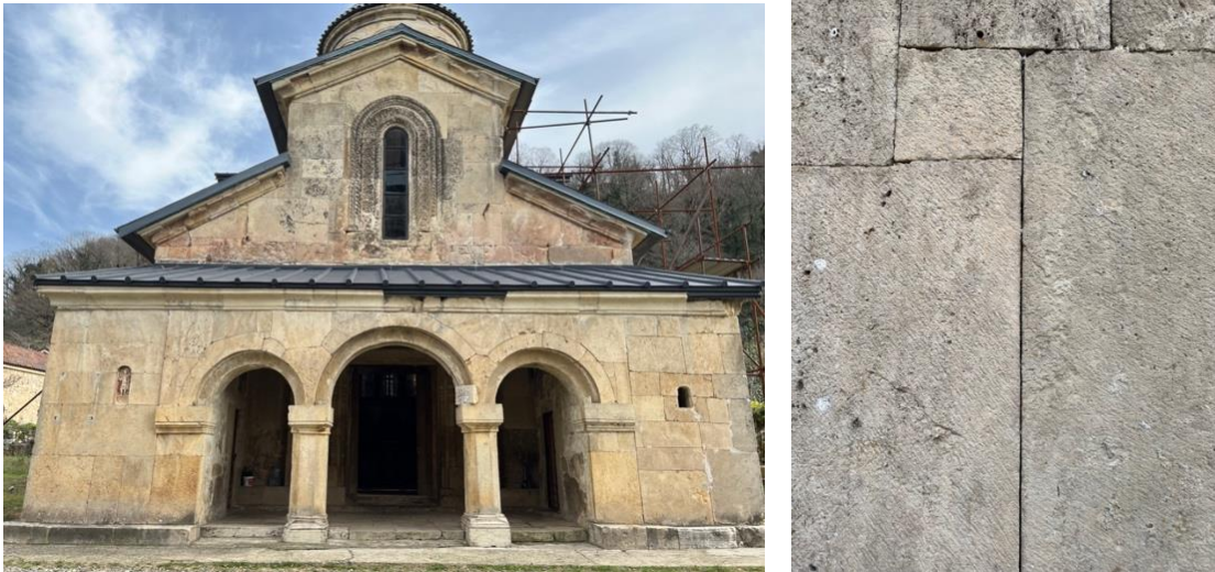
Fig. 58, 59. View of the façade of the Church of Saint George: need for infills in external stone joints, to avoid water penetration
