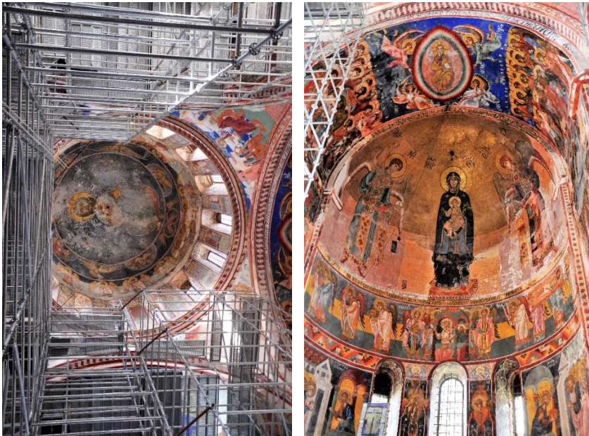
Fig. 36, 37. The scaffolding in the interior of the church: view to the cupola and to the altar
