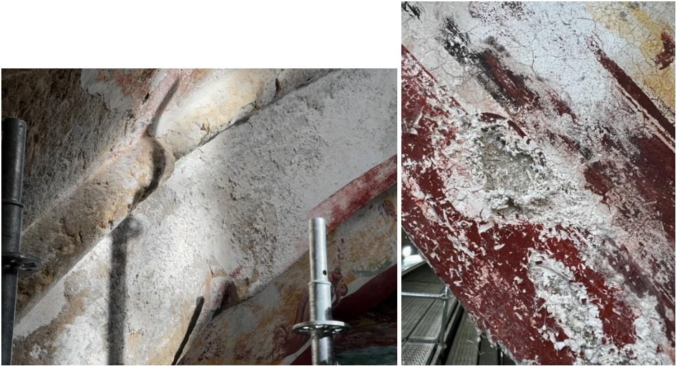
Fig. 32,33. Areas with severe plaster decay under the northwest pendentive
