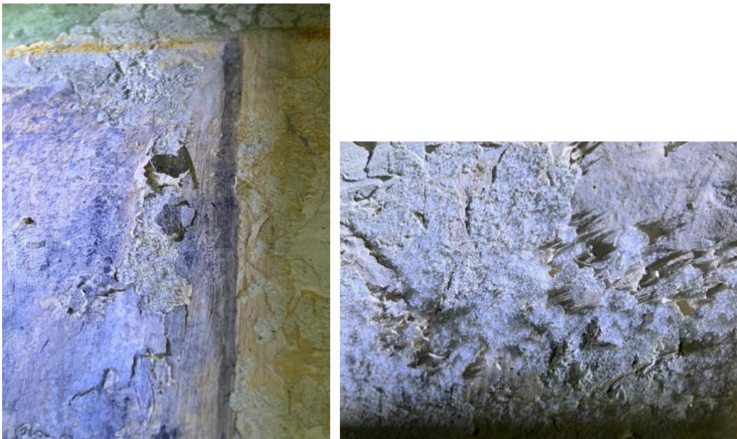
Fig. 29, 30. Detachment of paint layer and salt efflorescences in the northern wall of the west wing
