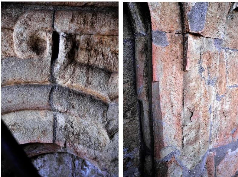
Fig. 53, 54. North arm – west façade: open joint cracks, fabric detachment and salt crystallization
