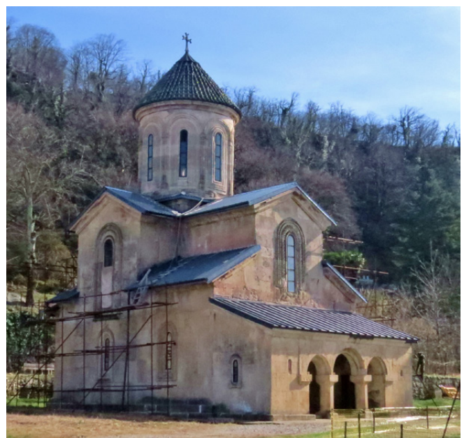
Fig. 2a and b: Roof cover of the St. George's Church, seen from the northwest, in June 2021 (Photo: Restruere 2021) and February 2022 (Photo: Europe Our House)
