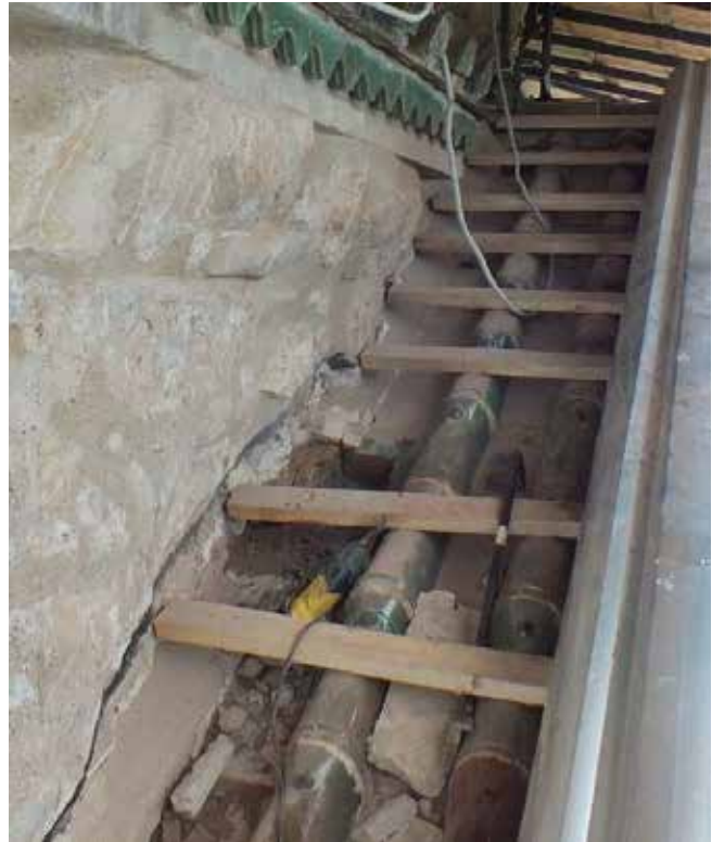
Fig. 4: Sondage R3. “From this sondage, it was possible to understand that the thickness of the mortar between the insulating layer and the tiles does not seem to be sufficient to ensure that the nails fixing the tiles do not pierce the insulating layer making the insulating layer ineffective.”
