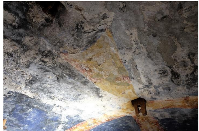
Figure 39: Points E and E', west wing vault, north side (efflorescence)
