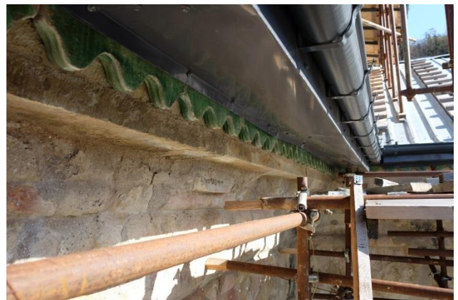
Figure 23: detail view of cornice and the eaves of a temporary roofing leaning against roofing tiles layer
