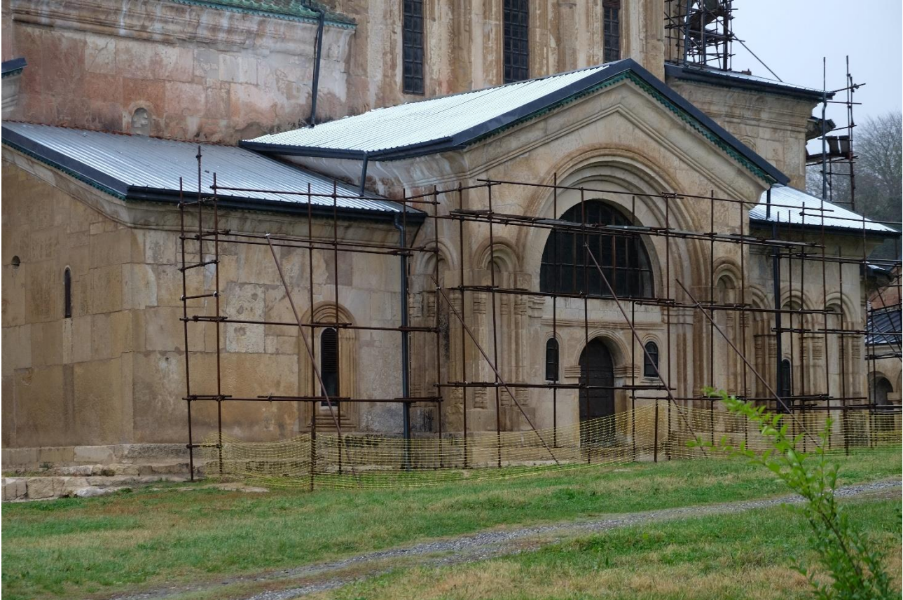
Figure 12: Church of the Virgin Mary, view of the south front with downpipes d4 and d5
