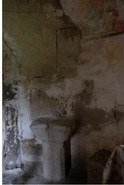
Figure 36: Point B, environment 6, north side of the apsidal hemicycle; point B', efflorescence
