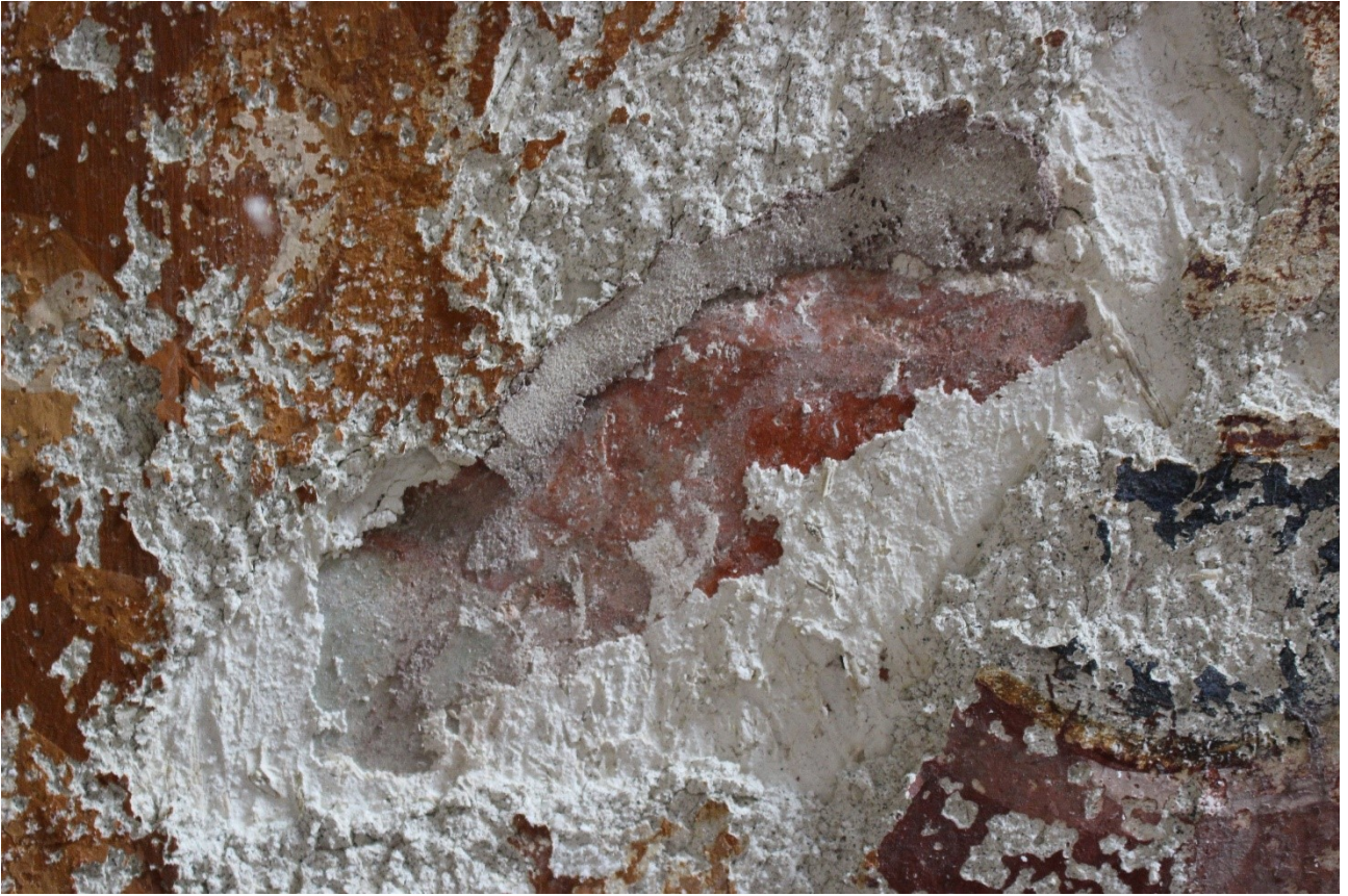
Detachment of portions of plaster due to the failure of the protections ( stucco curbs)
