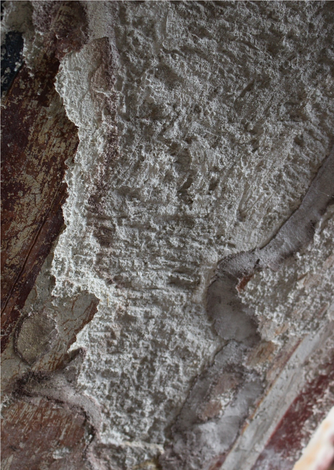
Detachment of portions of plaster due to the failure of the protections ( stucco curbs)
