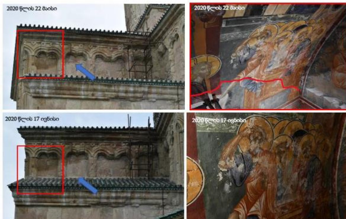
Photos: Upper part: May 22, 2020. Lower part: June 17, 2020. Exterior and interior parts of the south wall of the west arm.
