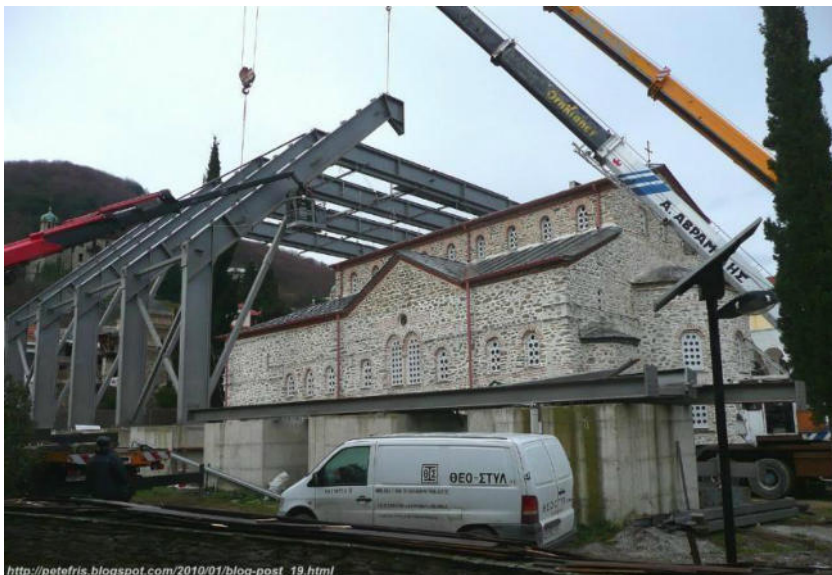
Fig.3. Protaton Church – Placement of reinforced inclined iron beams of protective metal scaffolding
