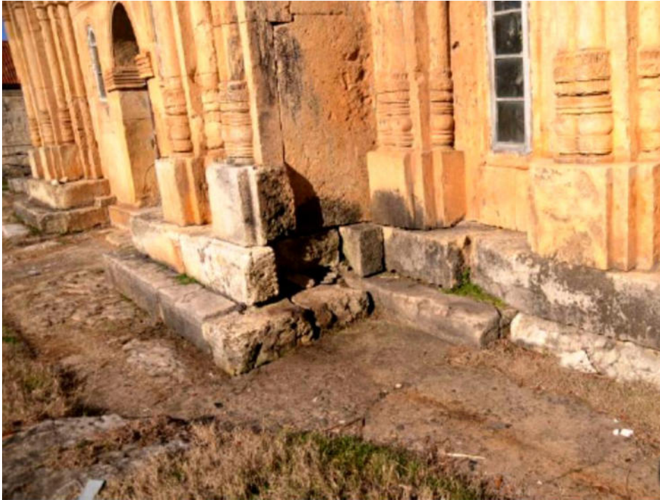
Fig.2. The crepidoma of the Church of the Virgin with the old drainage system around it (2015 joint ICOMOS/World Bank Advisory mission, fig.10)
