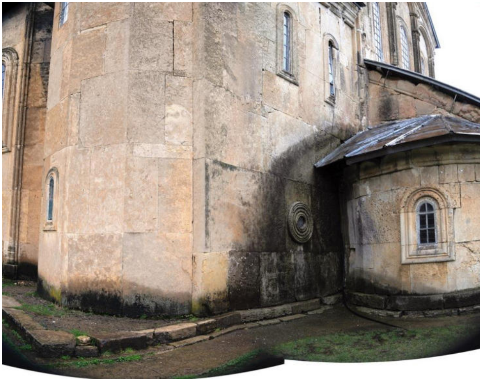
Fig.1. Descending and rising damp identified in the basement of the masonry of the Church of the Virgin (2010 World Heritage Centre/ICOMOS/ICCROM mission)
