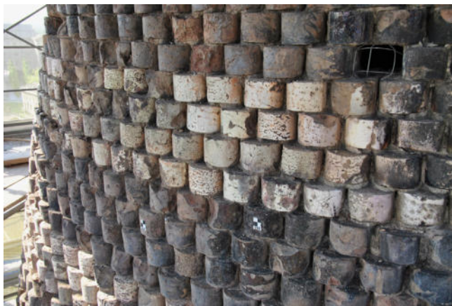
Fig. 2. Particular of the conic spire, realized with dichromatic glazed bricks: white and black. The masonry shows deterioration, cracks and erosion of the bricks.
