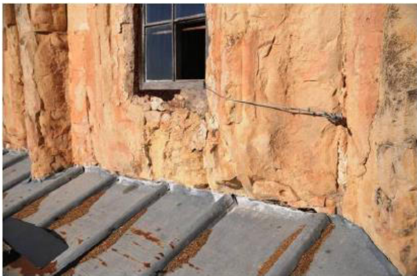
Facing masonry to the tin covering – existing condition (Fig.13 of the 2015 mission report).
