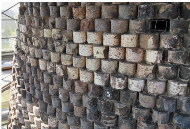
Fig. 2. Particular of the conic spire, realized with dichromatic glazed bricks: white and black. The masonry shows deterioration, cracks and erosion of the bricks.
