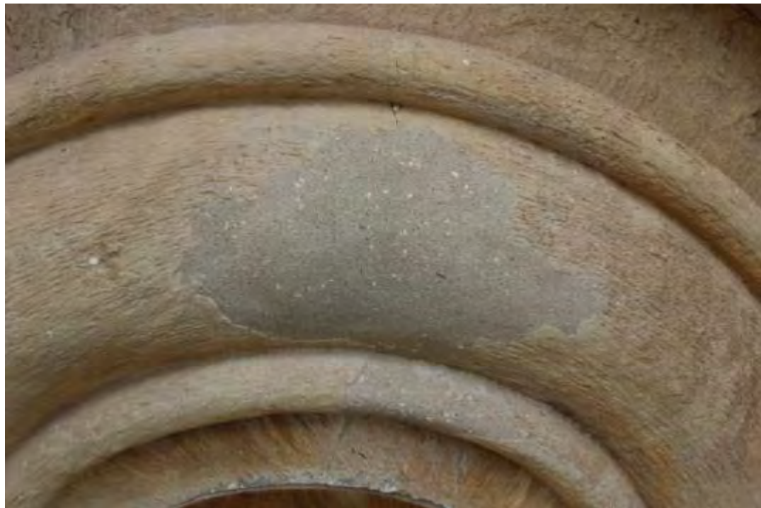
36-37. Consolidation of missed parts of masonry by lime and pozzolana, Drum Upper level
