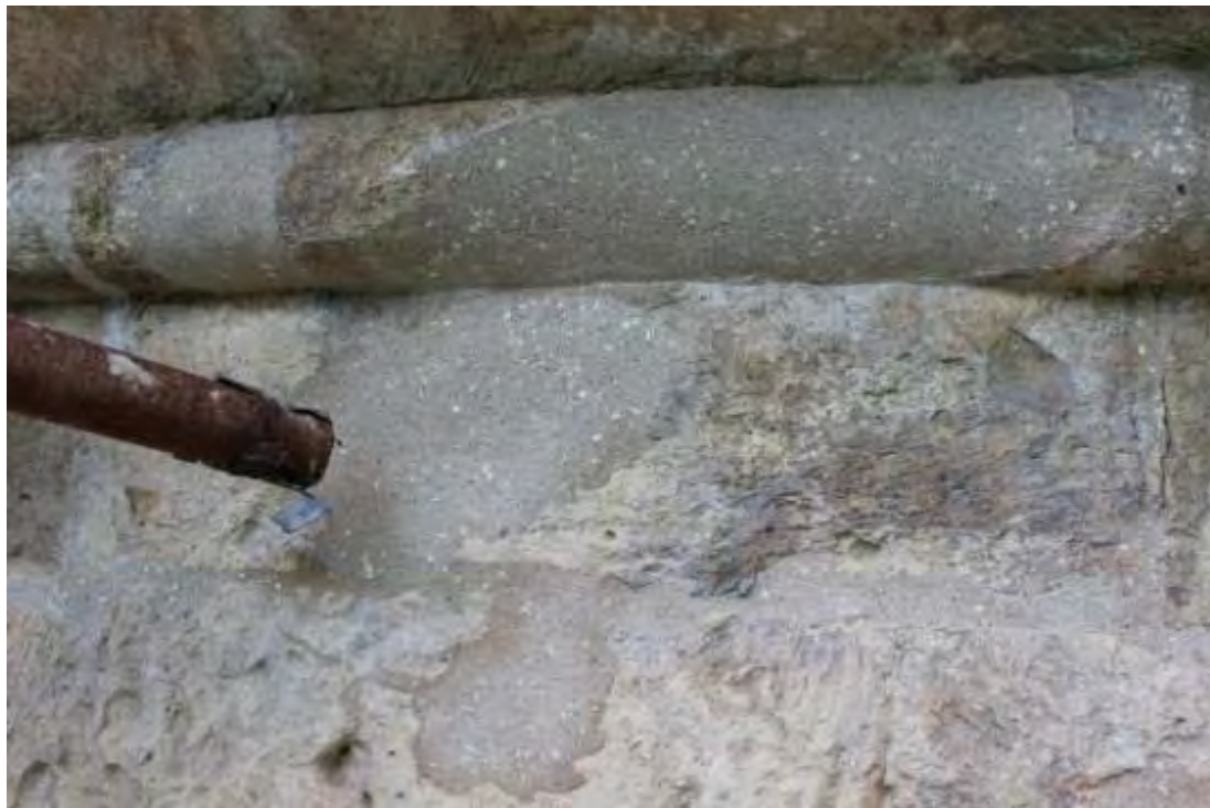
32-33. Filling of Joints & Consolidation of missed parts of masonry by lime and pozzolana, Drum Upper level, North-Western side
