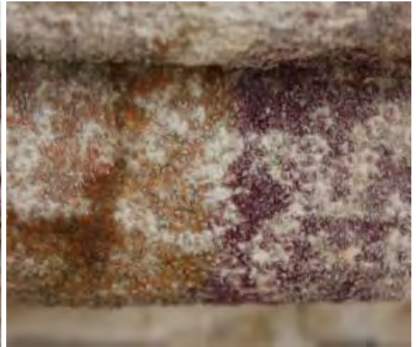
Fig. Biological damage
