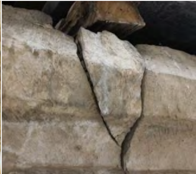
Fig. Stones damaged/ affected by rafters
