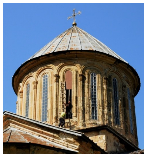
Fig. 18. The cupola : condition before hypothetical starting the architectural rehabilitation works
