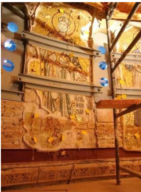
Figure 12. Steel elements to confine on two levels the masonry piers. Note the old I – beam on the lower part.
